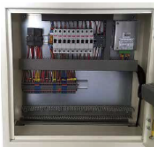
Automatic Control Panel
